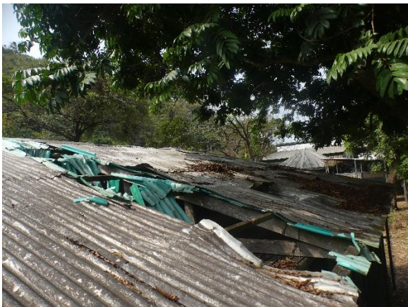
Image 21. View of the damaged roof above Western lowland gorilla Chella night den.
