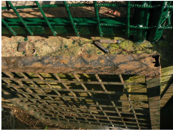
Image 21. View of damage sliding door (upper Drill satellite).
