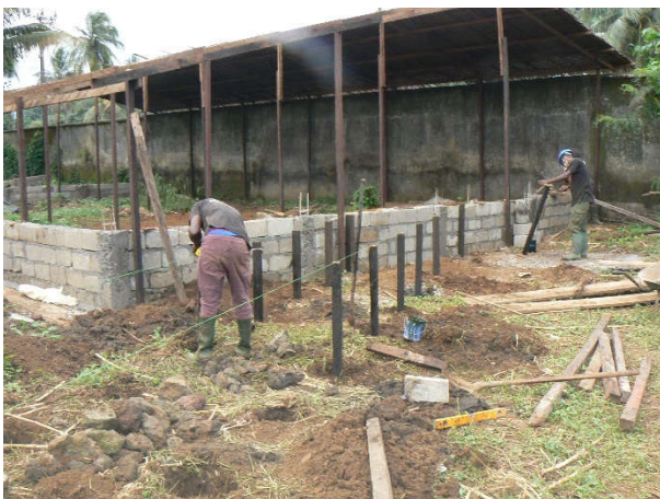
Image 13. Protective wall to prevent flooding of the composting area during the rainy season.
