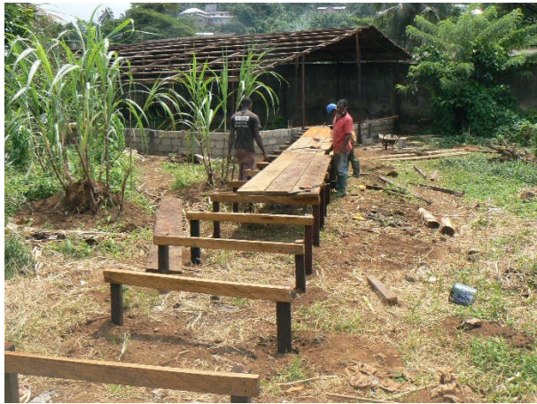
Image 15. Elevated wooden path installation to be used by the animal care staff to dispose of animal organic matter collected from the night dens.
