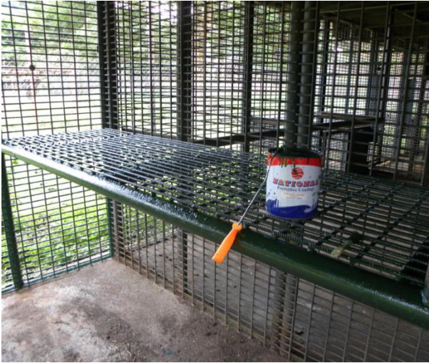
Image 22. Repaired and replaced mesh are painted with a rust-resistant paint to increase their longevity
