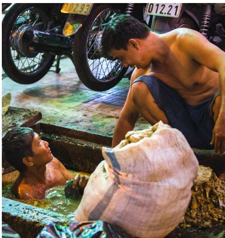
Two men cleaning the sewer at night on a street in Ho Chi Minh City, Vietnam © Shutterstock
