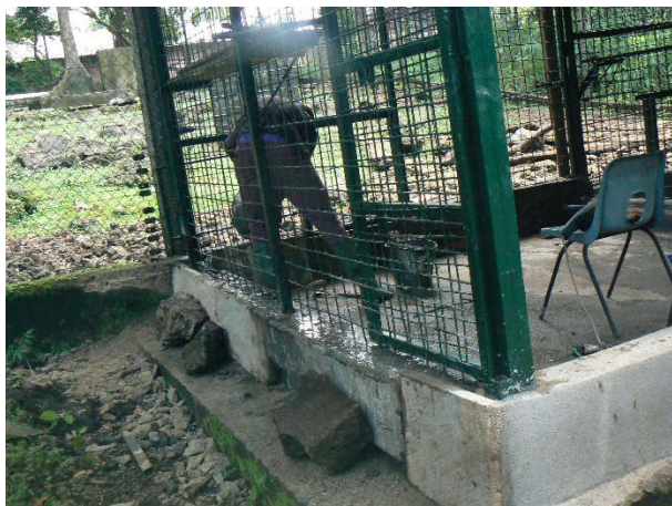
Image 24. Concreting and plastering of the foundation wall of the Mandrill satellite cage.
